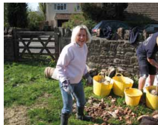
Tessa Munt MP lends a hand with Rodney Stoke lime mortar walling
